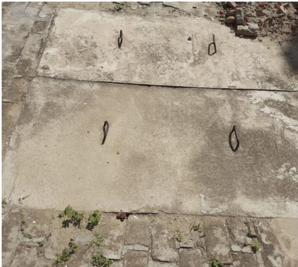
Rainwater harvesting pit
