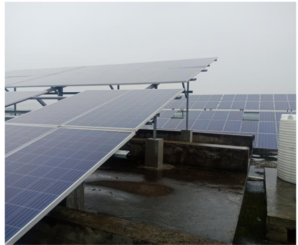
Solar PV installed on roof
